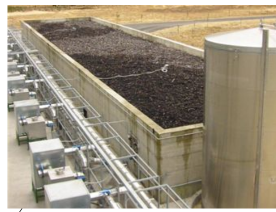
(3) BIOFILTER FOR THE ODOUR PROCESS AIR ABATEMENT
