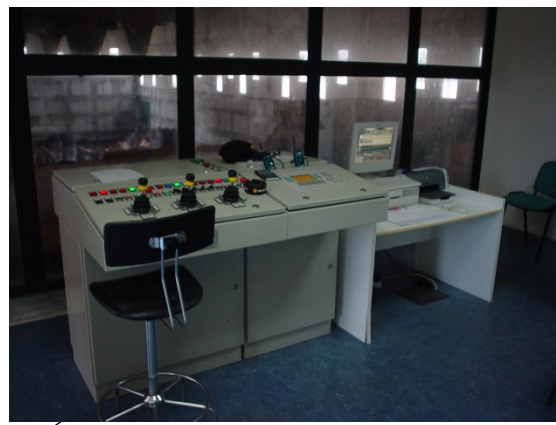
(2) CONTROL SYSTEM AUTOMATIC 24/7
